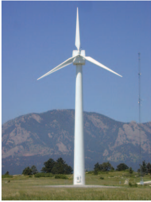
Northern Power 100kW turbine
