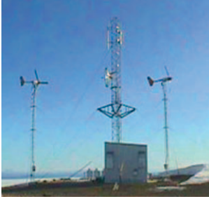
Bergey WindPower 1kW turbine on telecommunications station in Bristol Bay, Alaska
