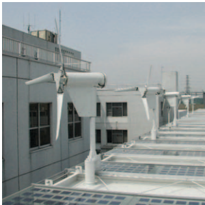
Proven Energy 2.5kW turbine rooftop array
